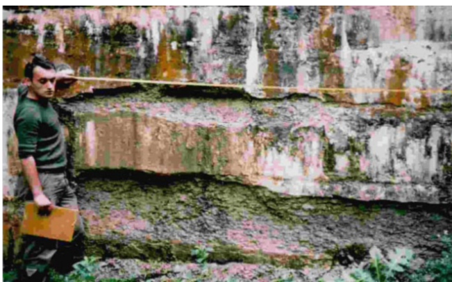
Figure 7 The dam 8B3,0 in Zimbrului Valley degraded by water and alluvia erosion in the area of the overflowed body (Photo: Clinciu 2003).
