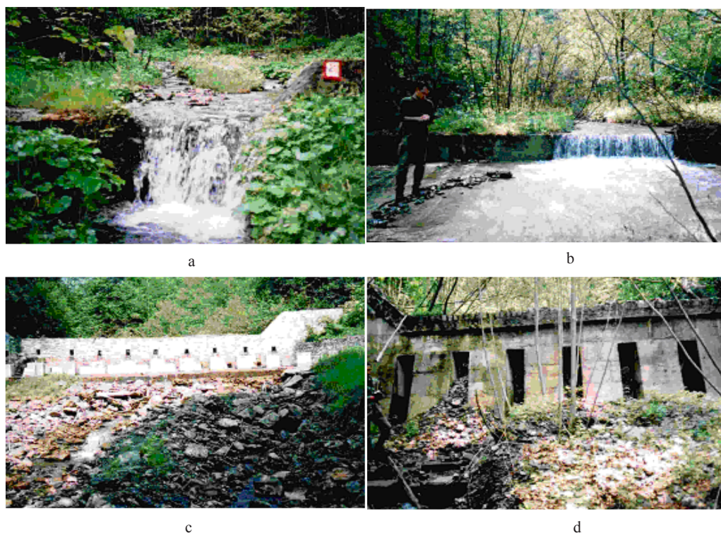
Figure 1 Torrential hydrographical management works in the Tărlung Valley at 20 (25) years from their construction
